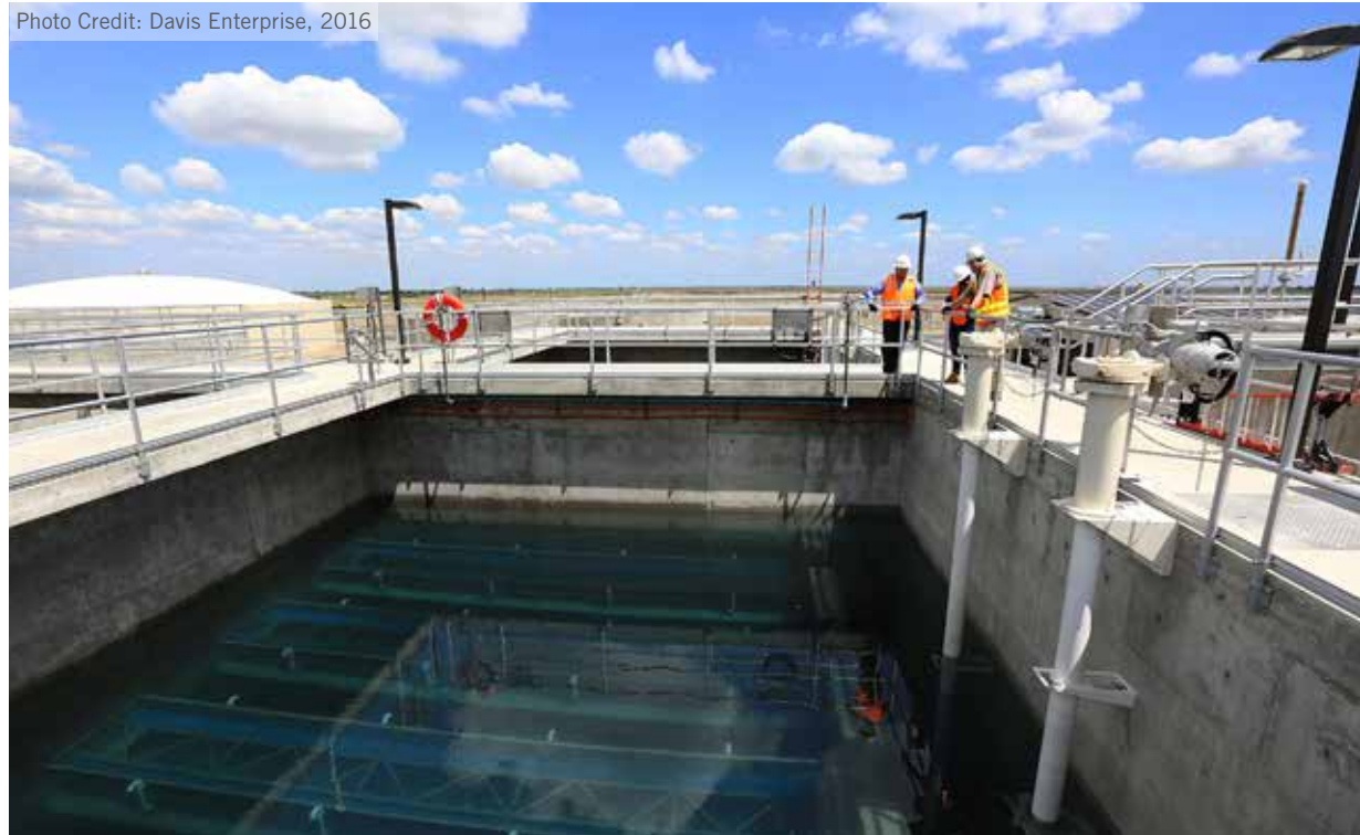
Woodland-Davis Surface Water Processing Station
