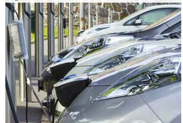
Figure 8.2.b: Electric Vehicle Infrastructure
